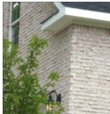
Brick with Weeping Mortar
